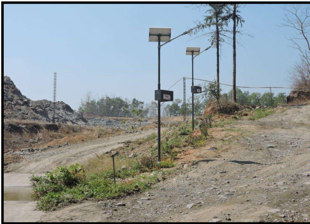
Solar light in the project site
